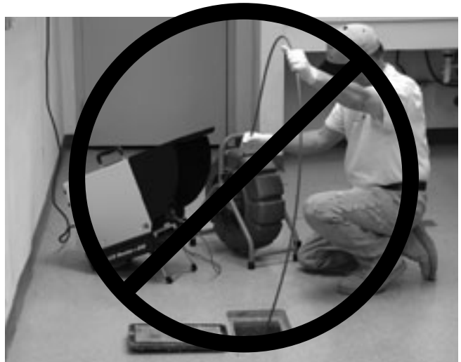
Figure 27 – Improper Cable Push
