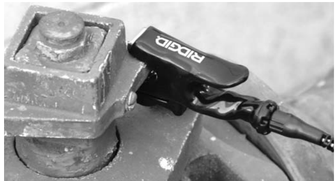
Figure 8 – Connecting Cable Lead To Target Conductor.
